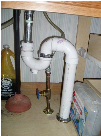
Sink drain has an improper trap — inspection view
