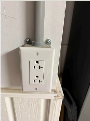
Shock protection is missing at these outlets — inspection view
