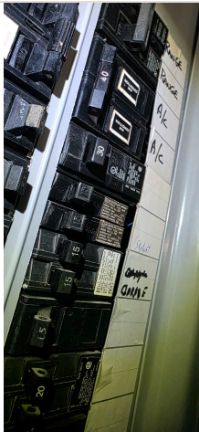
Improper breaker fit visible — inspection view
