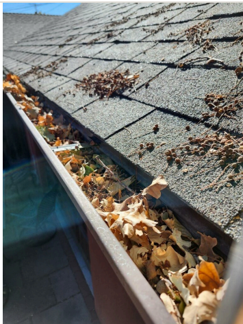
Debris accumulation — inspection view
