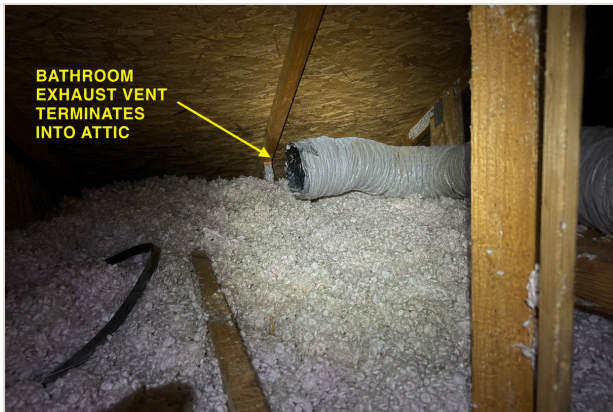
Bathroom exhaust duct terminating in the attic
